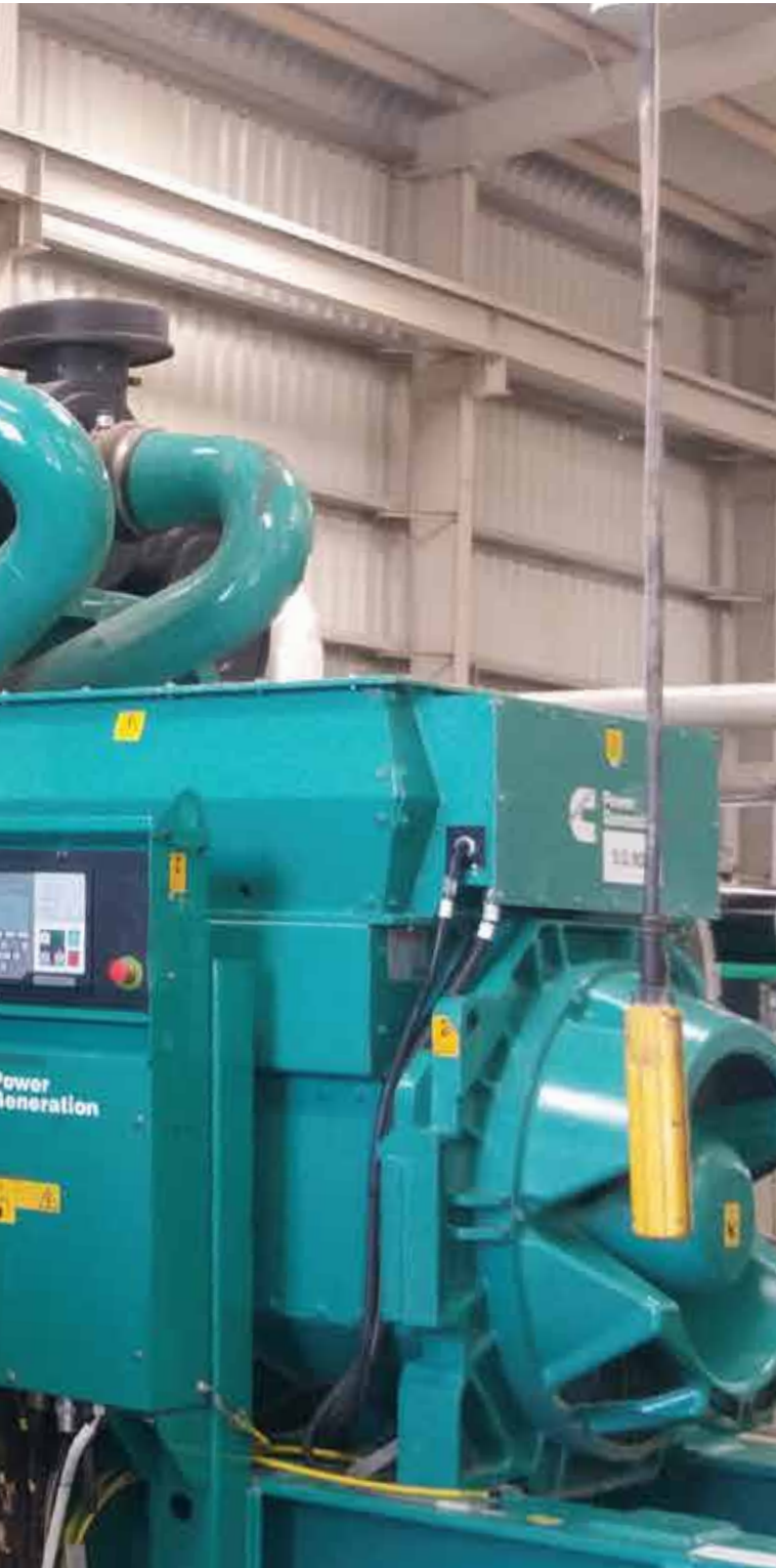
MAZOONA POWER STATION
